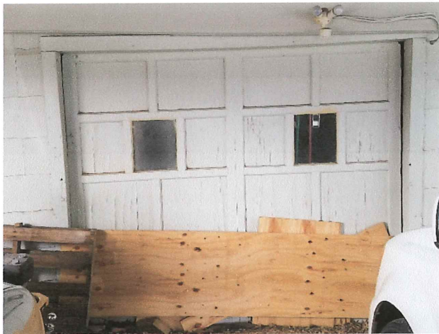
Inoperable garage door.
