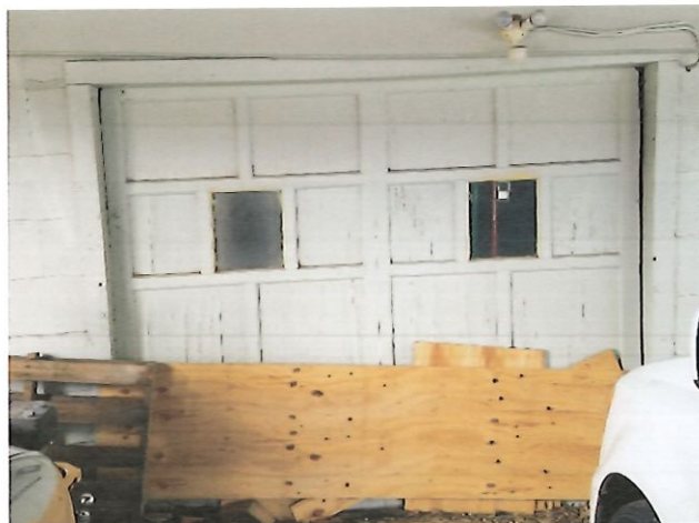
Inoperable garage door.
