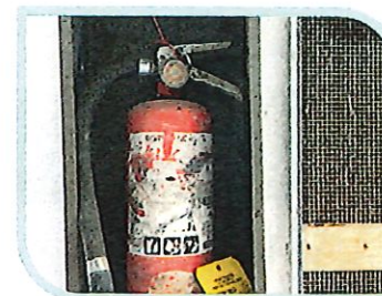
Fire Extinguisher Violation
