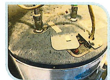
Improper Water Heater Installation
