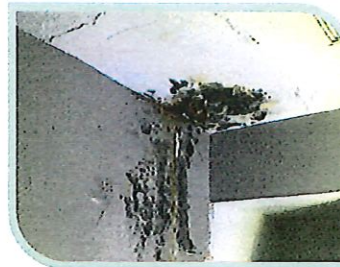
Damaged Interior Surfaces
