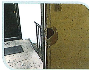
Damaged Interior Walls
