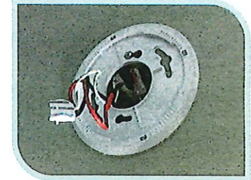
Missing or Damaged Smoke Alarm
