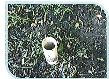
Missing Cap on Clean Out
