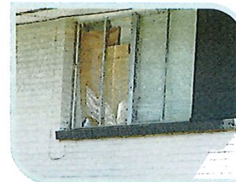
No Screen/Broken Windows
