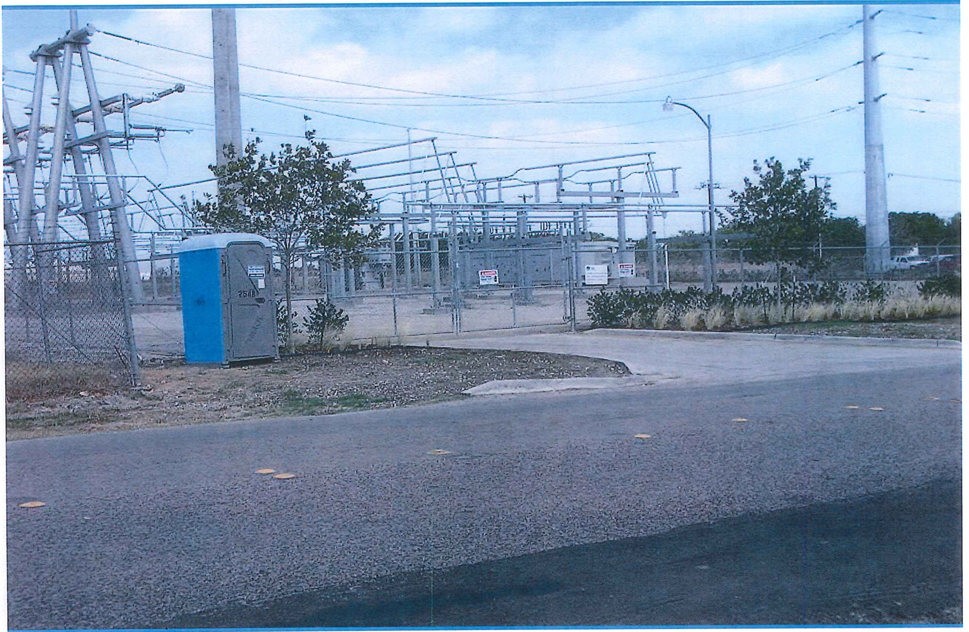
Carrollton Country Club substation
