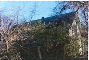
s in roof.west side.20160113_0
