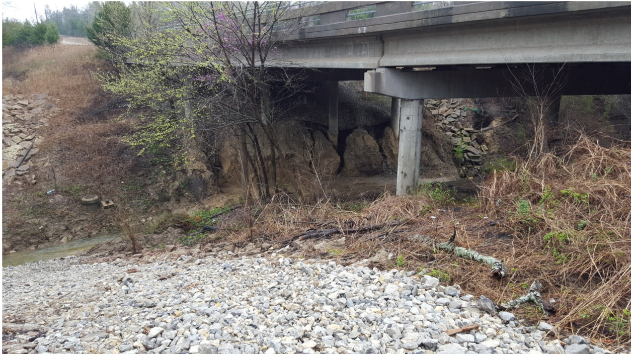
Fallon Bridge Erosion Control – Before
